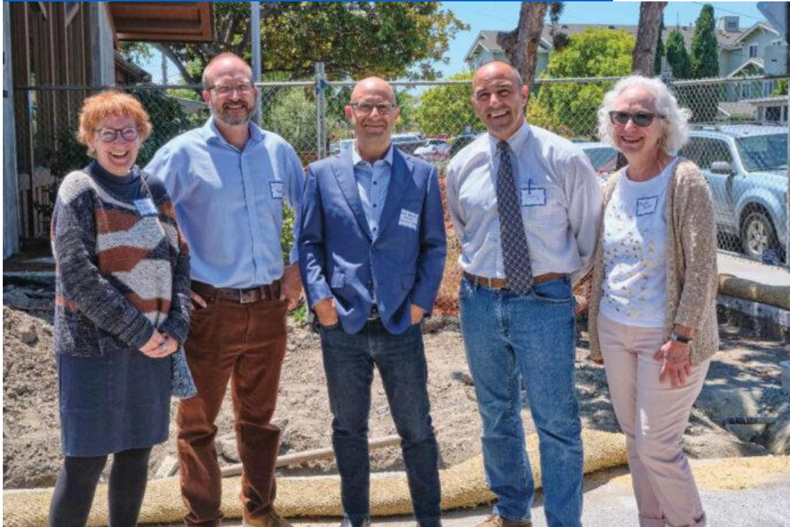
Friends of the Santa Cruz Public Libraries President Janis O'Driscoll (from left to right), SCPL Deputy Director Eric Howard, Architect Abe Jayson, Congressman Jimmy Panetta, and Committee Chair Martha Dexter at Branciforte Branch Construction Site. — Courtesy of FSCPL
