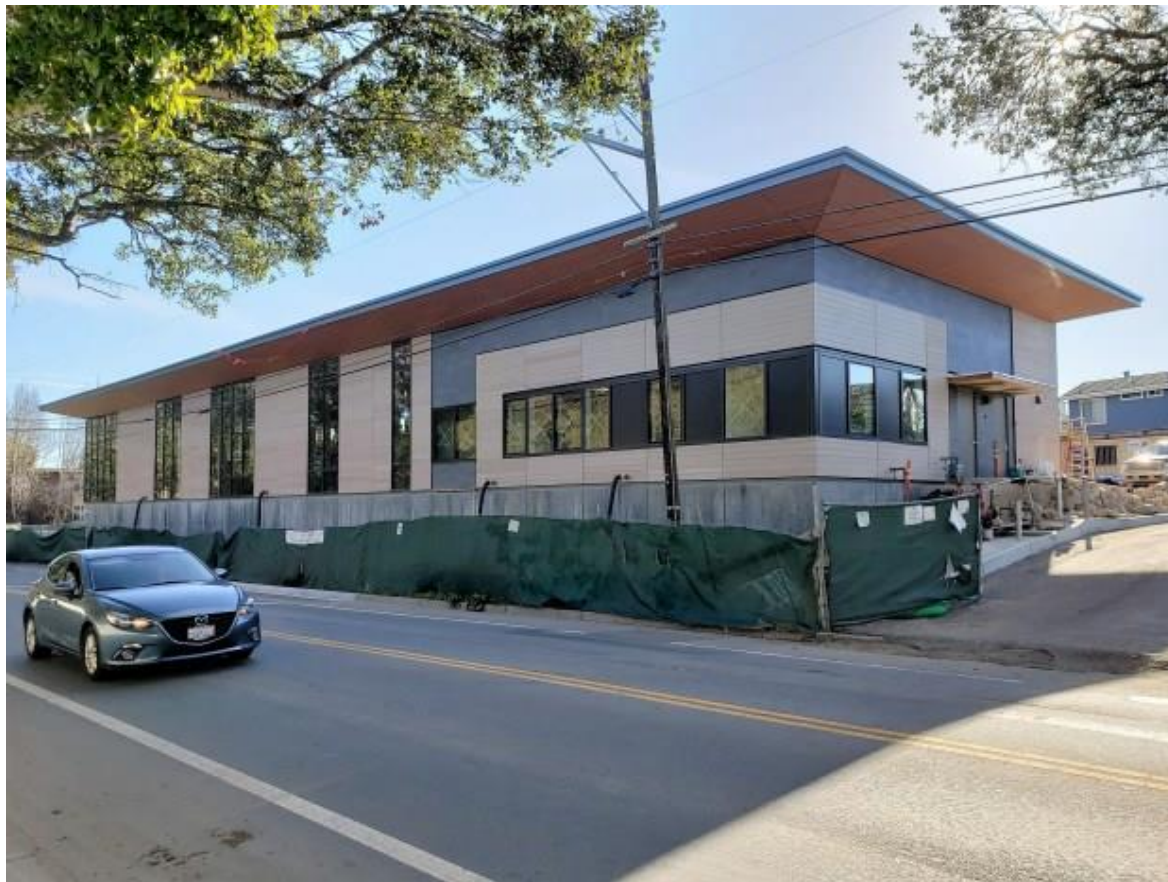
Work continues on the new library in Capitola on Feb. 26. (City of Capitola — Contributed)
